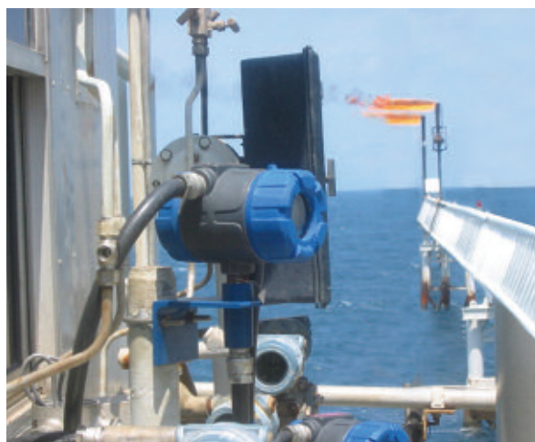
Due to environmental laws and restrictions, oil and gas platform operators must monitor and report the amount of flared gases. The consistent composition, low flow sensitivity, and high turndown capabilities make the TA2 an ideal flow meter for this service.
