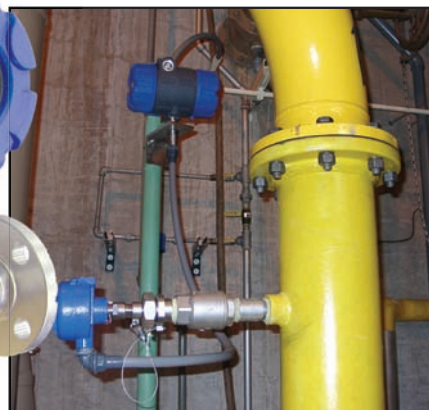
FIGURE 9. A thermal mass flowmeter with remote electronics is used to measure the biogas flow from an anaerobic digester. The probe is located roughly 3 ft from the floor, and the remote head permits the operator to view the display. A retractable probe assembly is used to permit the removal of the probe from the pipe to ease maintenance while minimizing leakage of a combustible gas
